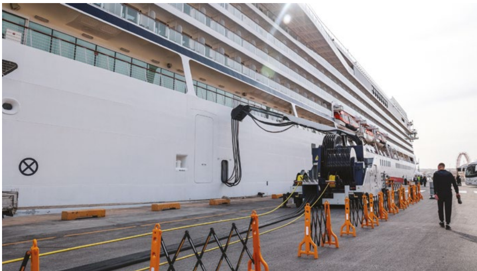
Infrastructure Malta, Shore to Ship - Onshore Power Supply
